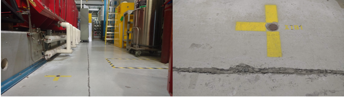
Figure 19: Evidence of floor slab stress and potential shifting in the ISAC-I experimental hall.
