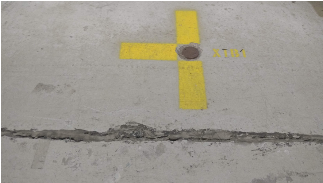
Figure 12: Top: Crack in the ISAC Experimental Hall floor, running parallel to the RFQ. The crack developed in what was originally a concrete floor joint. Bottom: close up of the crack, showing its extent and presence of weathered caulking.
